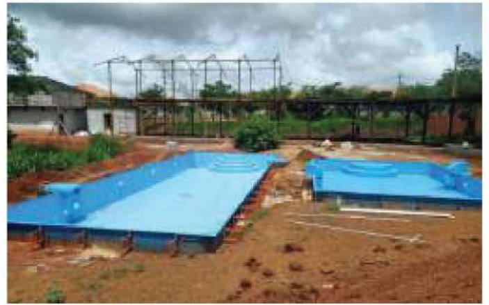
WATER PARK POOLS, 3 POOLS,KARNATAKA
